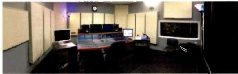
The new audio control room at Twin Cities Public Television’s renovated headquarters includes a Calrec Omega console and extensive RealTraps acoustic treatment.
