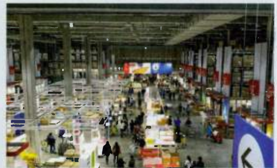
A new IKEA store in Goyang, Korea sports a sizable Community pendant loudspeaker system.
