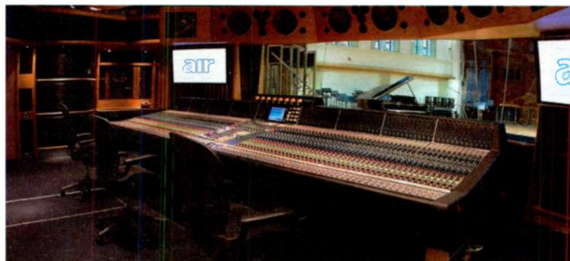
Lyndhurst Hall control room
