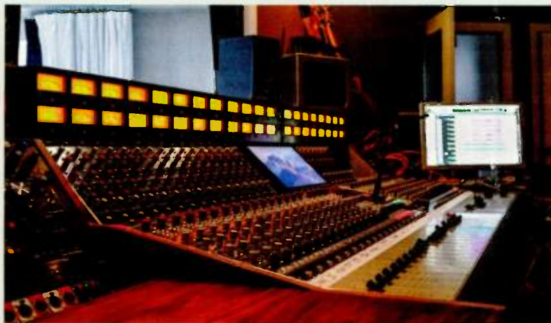
The mixing desk is a 40-input Rupert Neve Designs 5088, fitted with 24 mono input channels and 24 Shelford 5052 mic preamp/EQ modules, plus eight additional stereo input channels.
