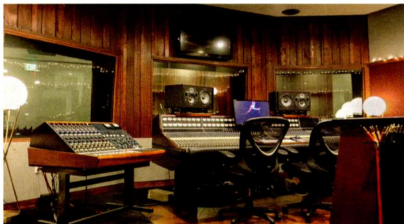
Control Room A offers a hybrid approach, making use of a 48-channel API Legacy Console and vintage Neve BCM10 sidetar, along with outboard gear from manufacturers including Shadow Hills, Pultec, Empirical Labs, Universal Audio and Tree Audio.
