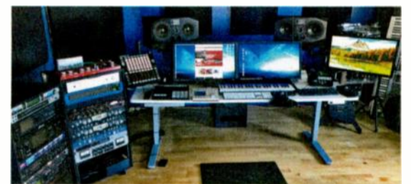
Bruce Somers reduced cable clutter in Undercurrent, his multistory studio, by implementing a Dante-enabled RedNet network.
