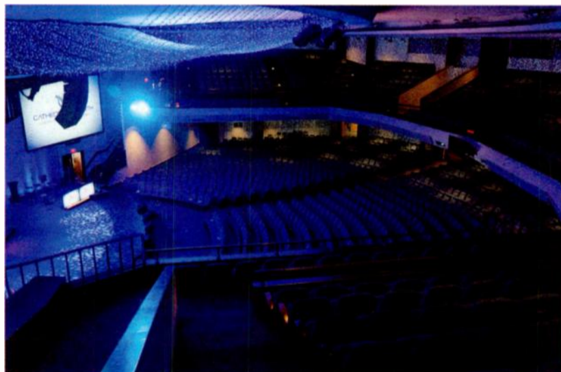
Sound Image installed a new audio system based around Martin Audio WPC line arrays in Cathedral of Faith.
