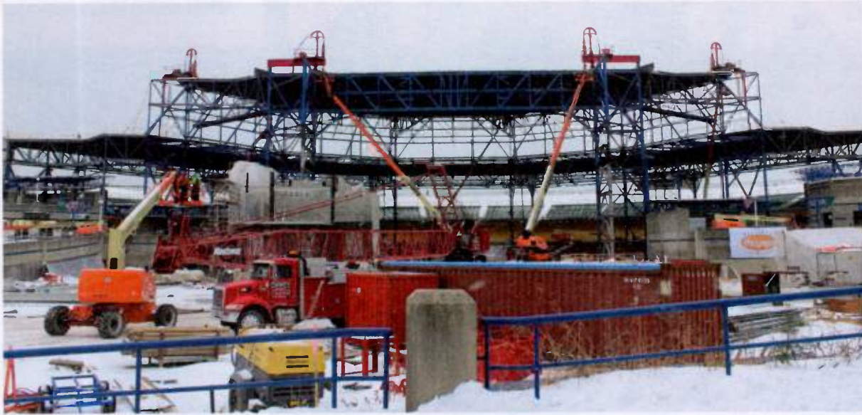
The 607,000-pound roof of the 23,500-seat American Family Insurance Amphitheater was raised 26 feet in one snowy day.
