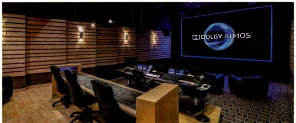
DAP worked with FM Design, Avid and Meyer Sound to update the facility.
