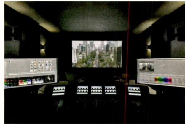
The new facility will house eight Dolby Atmos-certified stages and cutting rooms.
