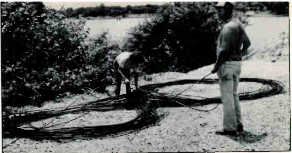
Fiberoptic cable is placed in a large figure-eight for the next pull. Thinner cable will form much more compact figure-eights.
