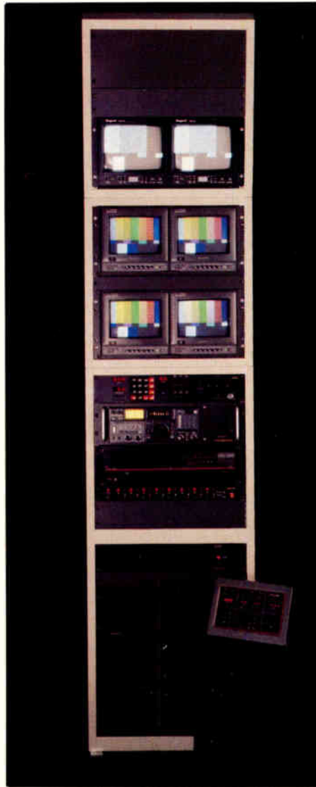
"FIGS" and "ROSE" control room for security room.
