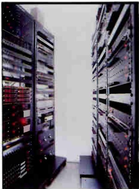
Equipment racks used at the installation.
