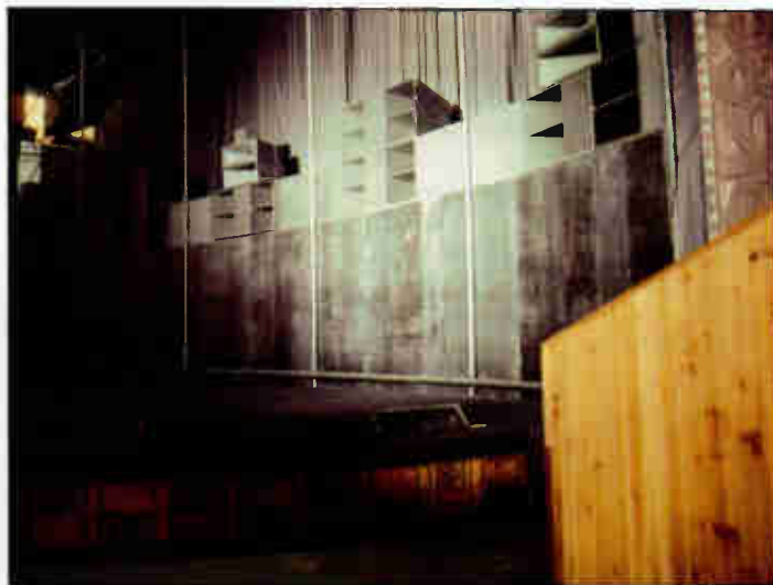
This shows the behind the screen HPS-4000 speaker compliment for a Showscan installation.
