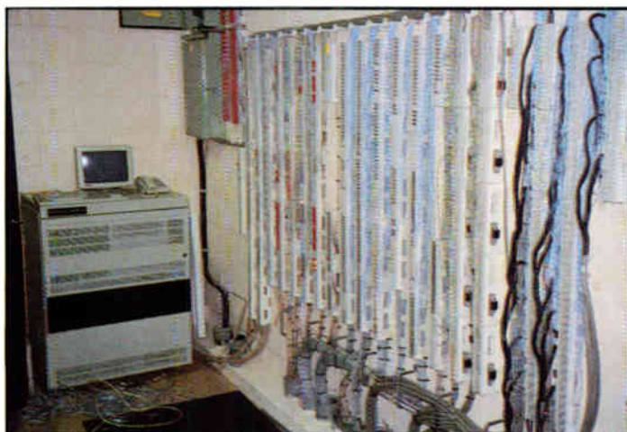
Installation at Buena High School in Sierra Vista, Arizona by Chambers Electronic Communications. Included in the install were Rauland Borg's Telecenter IV Plus and a Blonder Tongue RF distribution system. The photo shows the terminal boards behind the racks.
