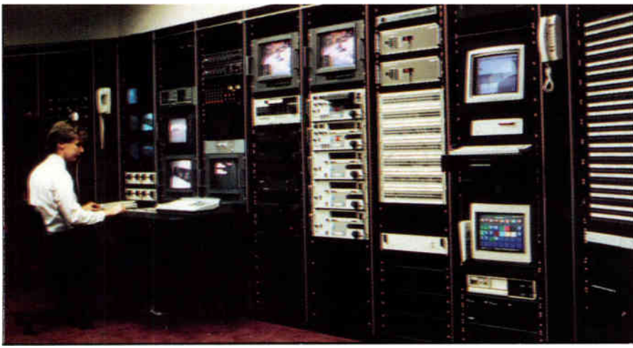
The control room at the University of North Carolina with its centralized scheme of program sources as installed by Acentech.
