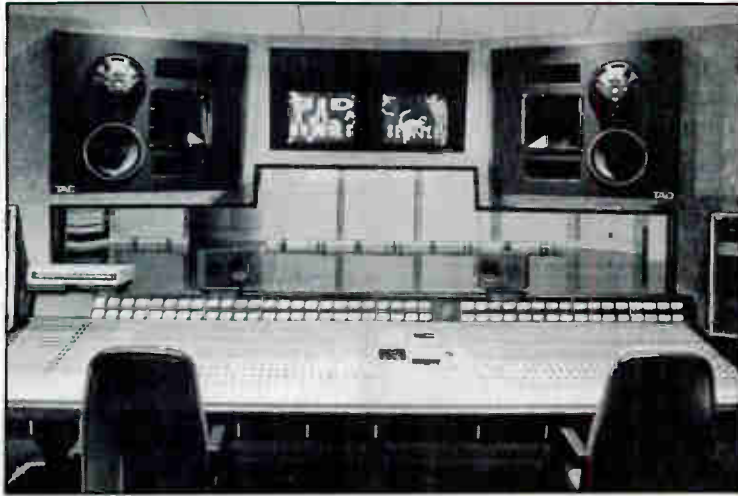
TAD studio monitors housed in more than 40 cubic feet of poured concrete.
