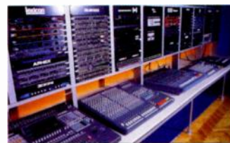
One side of the switcher-equipped recording room.
