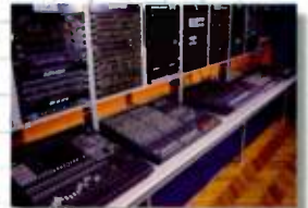
One side of the switcher-equipped recording room.
