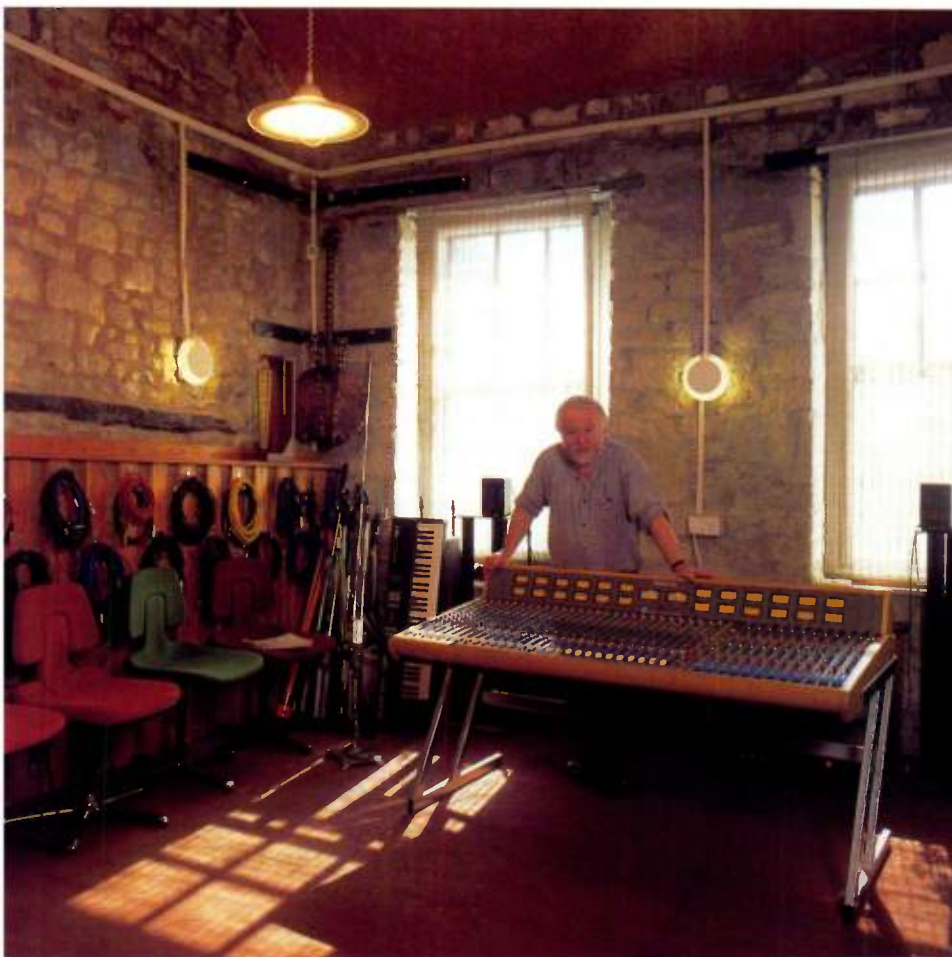
Terra Incognita's recording room, where David's Trident Series 65 mixing desk is awaiting installation in the control room.
