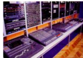
One side of the switcher-equipped recording room.
