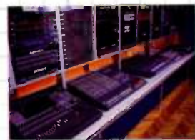
One side of the switcher-equipped recording room.
