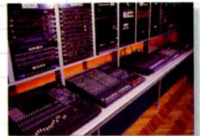
One side of the switcher-equipped recording room.
