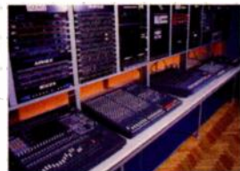
One side of the switcher-equipped recording room.
