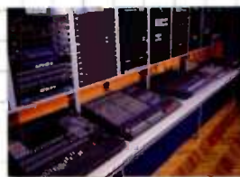
One side of the switcher-equipped recording room.
