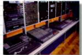
One side of the switcher-equipped recording room.
