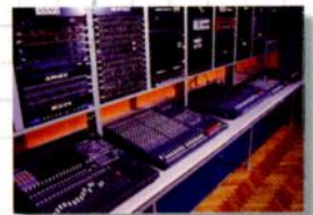
One side of the switcher-equipped recording room.
