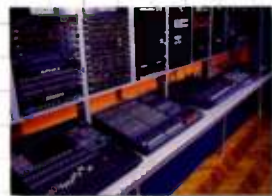
One side of the switcher-equipped recording room
