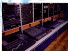
One side of the switcher-equipped recording room.
