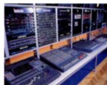
One side of the switcher-equipped recording room.
