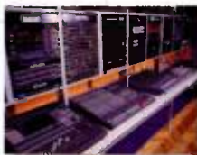
One side of the switcher-equipped recording room.
