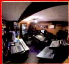
Dedicated room for studio monitoring
