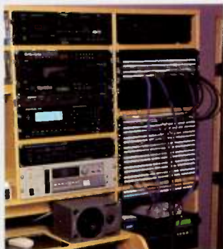
Installing balanced patchbays (as opposed to unbalanced ones) makes dealing with hum much, much easier.
