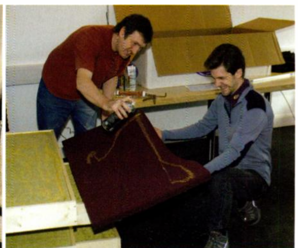
The foam panels go on top of the rockwool, secured with spray adhesive.
