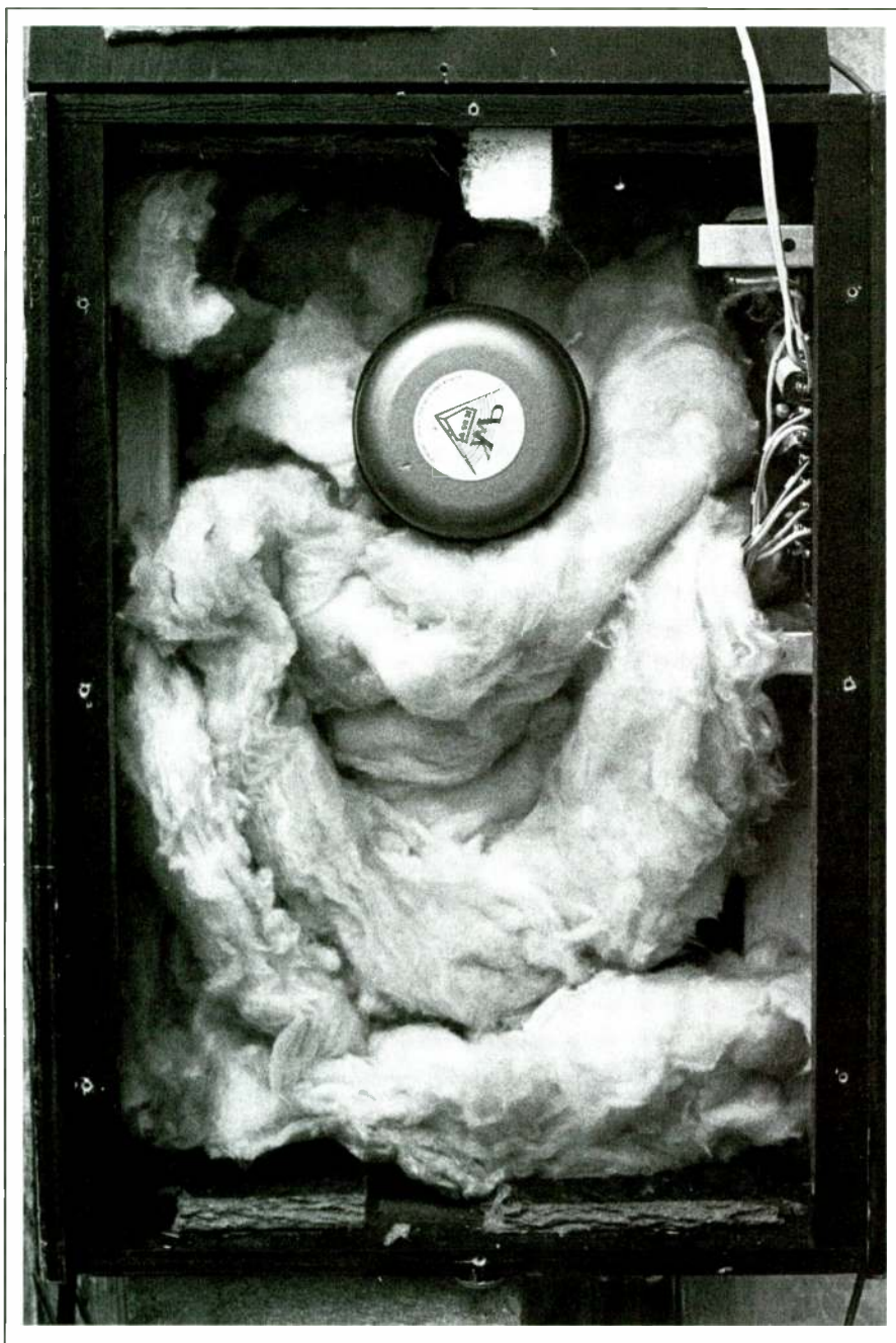
PHOTO 3: The fiberglass insulation is bunched in the center of the cabinet, where it is most effective.
