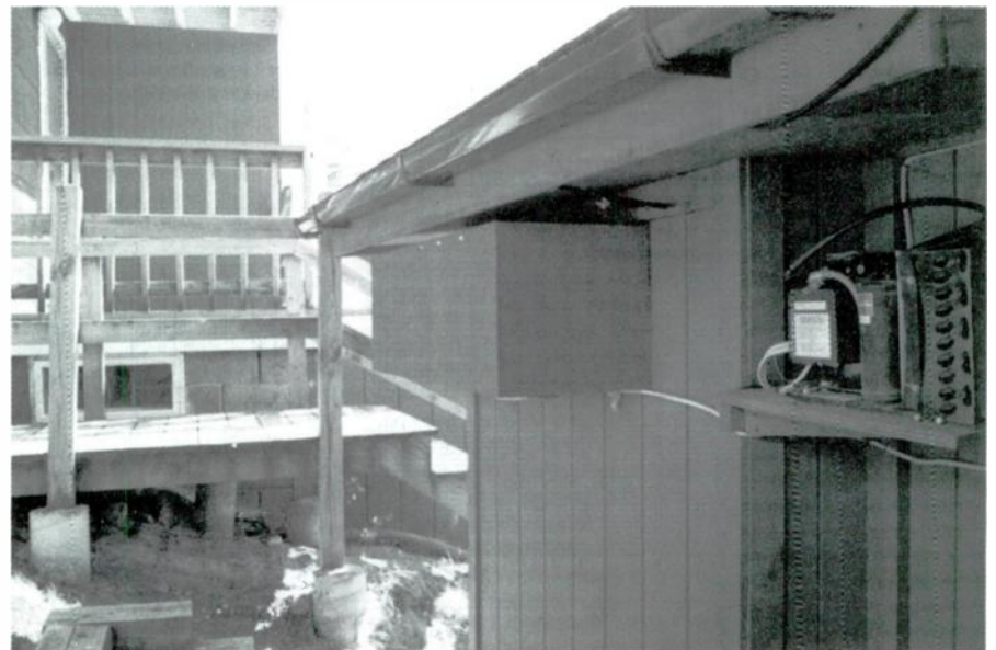
PHOTO 2: A subenclosure in place on a building rear wall.
