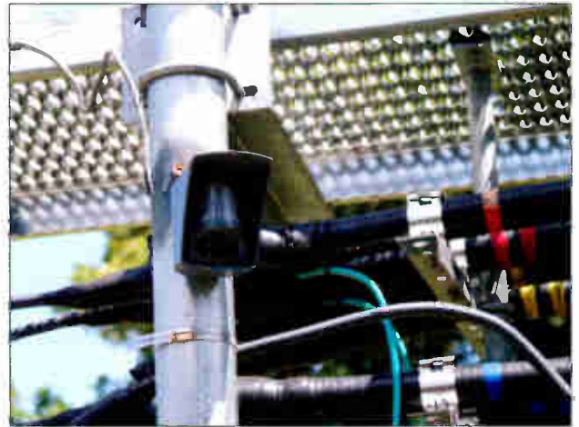
This camera gives a straight view from the cable tray looking outward, revealing any possible intruders to viewers at the security monitoring center. Metal thieves might be attracted by the copper in the wires shown here covered with green insulation.
