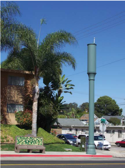
An SCI light pole with a decorative radome for a T-Mobile distributed antenna system in San Diego.
