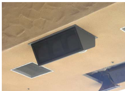
At a racetrack, an SCI Fibercell panel with low RF loss conceals AT&T distributed antenna system antennas in an enclosure made to look like a speaker box.
