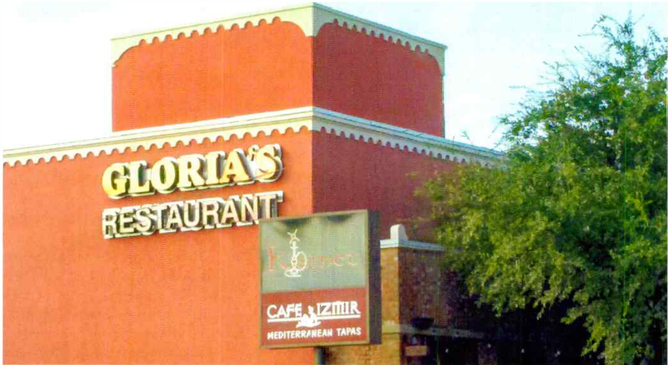
To conceal a Verizon Wireless antenna installation at Gloria's Restaurant on Greenville Ave. in the art district of Dallas, where no towers over 30 feet high are allowed, St. Charles Tower designed an artistic partition on two sides of the roof with the same scalloped cornice work along the top edge.
