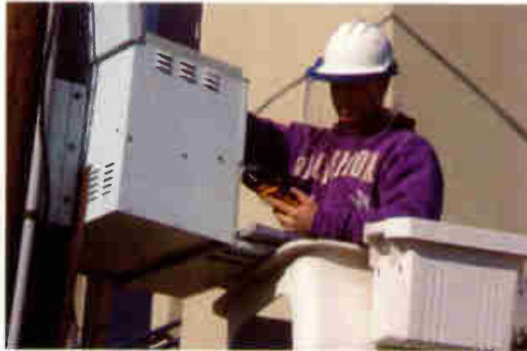
Wearing the required safety equipment, a technician tests the operation of an aerial standby power supply.
