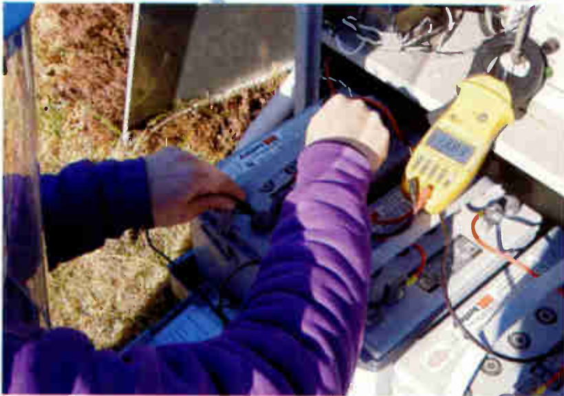
A technician measures individual battery voltage to verify proper voltage levels.
