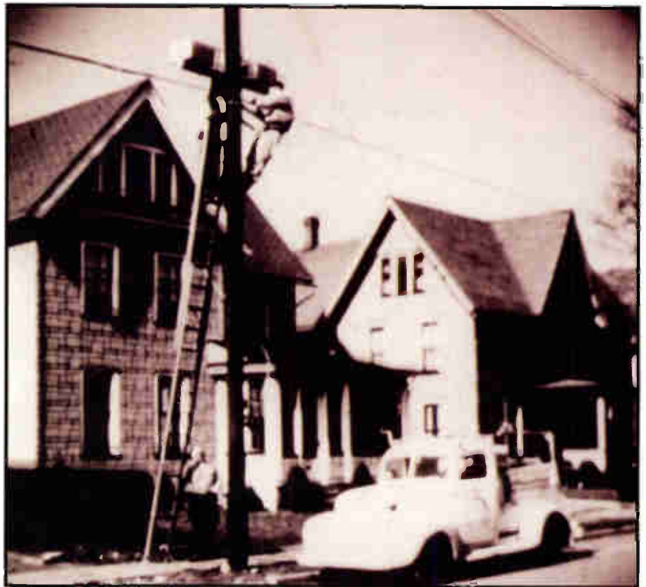
Some things don't change much: Laddercraft and pole-climbing are still staples in the industry, just as they were back in the early '60s.
