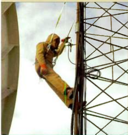
Danger averted by standing on tower rung.
