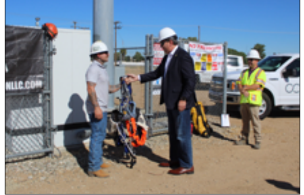
Tower Technician Dylan Pontes from JHC Construction LLC talks about all of the features of his climbing safety harness with Congressman Jay Obernolte during the visit to the Crown Castle tower site in Hesperia, California.
