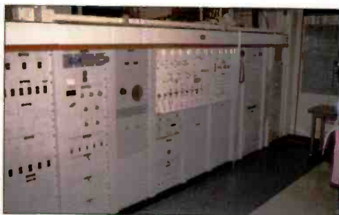
Three Collins 821A1 transmitters were used at the VOA site.
