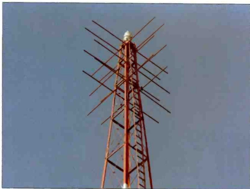
Detail of the top loading used on the towers.
