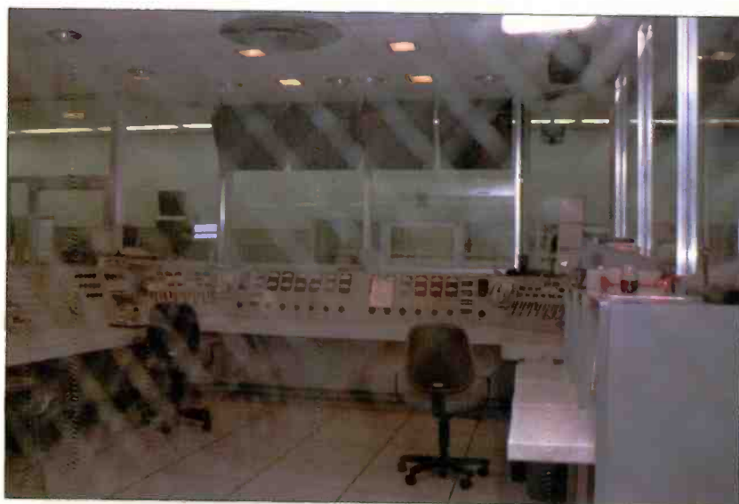
The transmitter control room.
