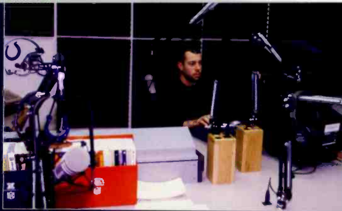
Indianapolis Colts Programming and Production Manager Chris Owens gets the feel of his brand new AirWave Broadcast Console from Harris Pacific in the Colts' new Harris-installed studio.
