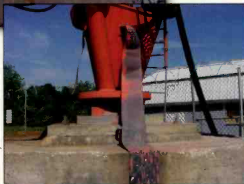
Examples of a poor tower ground (top) and a good tower ground. Not only is the conductor in the poor example too small, it is not attached.
