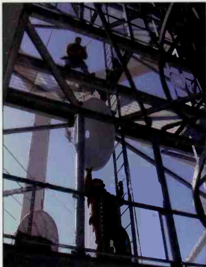
WNYC installed a full-power facility at Times Square.
