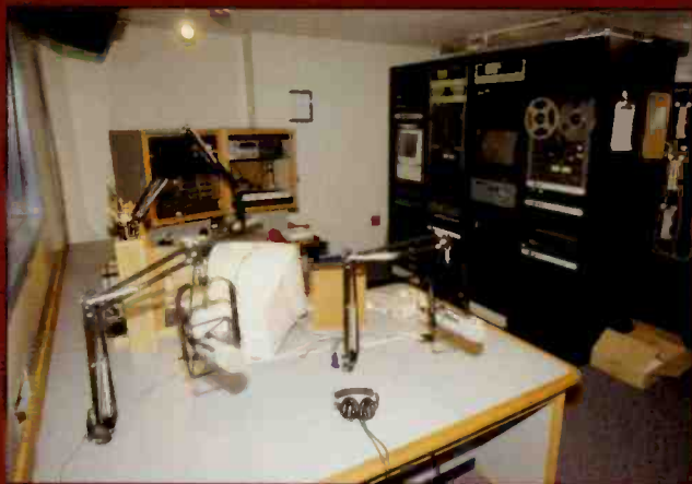
The Master Control Room/On-Air Room, has all necessary equipment placed within easy reach of the show host.
