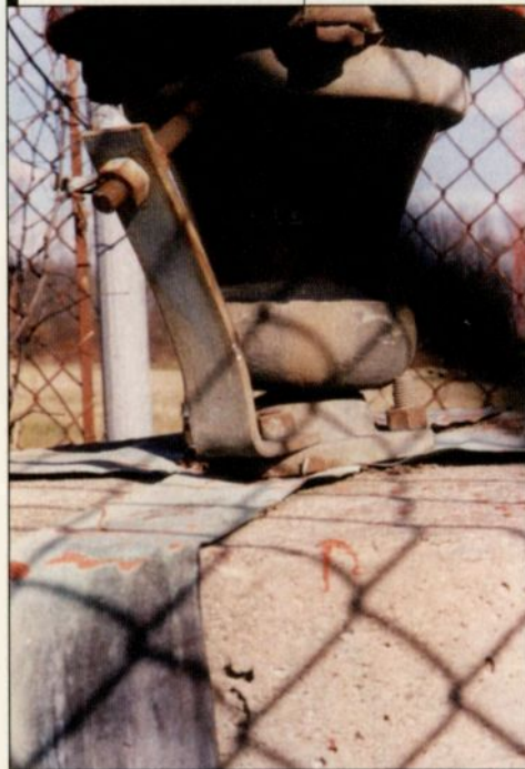
Physical changes, like this shifted tower base pier, can easily influence a directional array. Photo by Tracey Liston.
