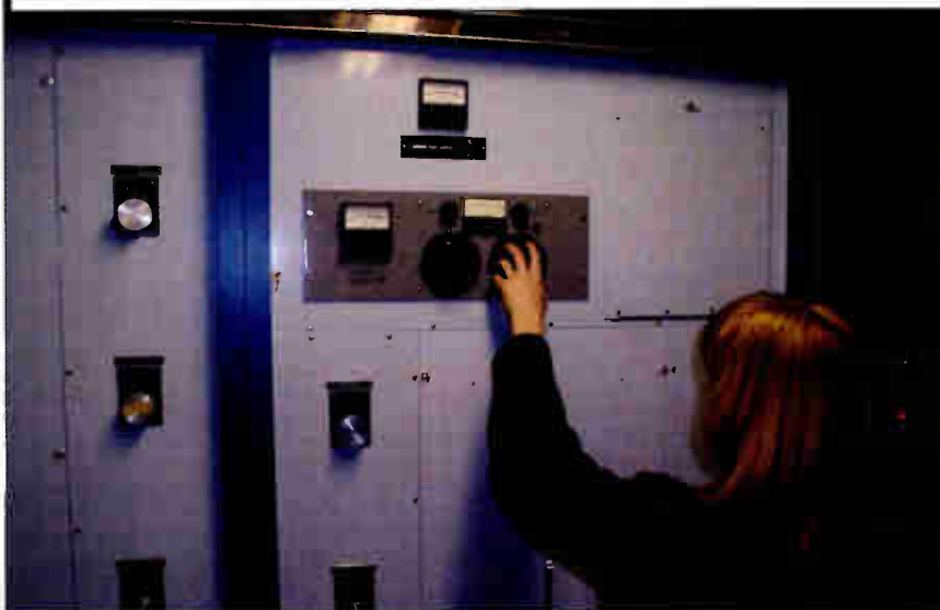
An OIB is a vital piece of equipment for a directional AM station and can be used to quickly diagnose antenna system operating problems.
