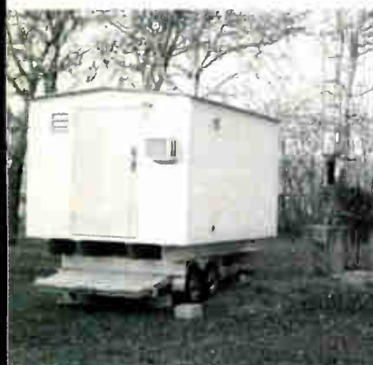
WCBS/WFAN Aux Tower New York, NY
