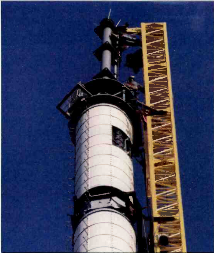
Workers set the channel 68 Andrew Trasar Antenna to the top of the tower. The workers are leveling it while it is supported by the ginpole. This antenna is the final piece of the tower. Photo by John Lyons.
