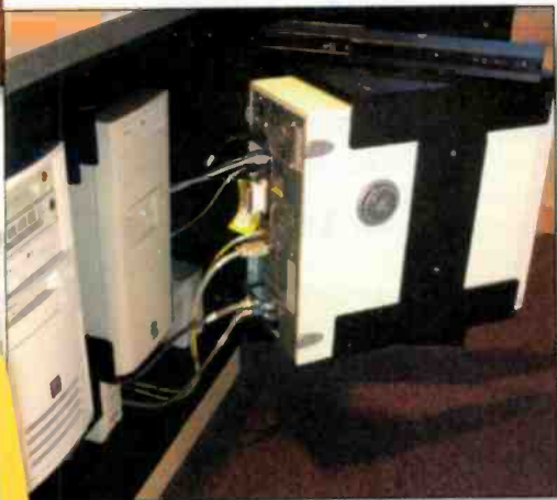
Access to the studios computers is facilitated by the mounts installed inside the Mager furniture.
