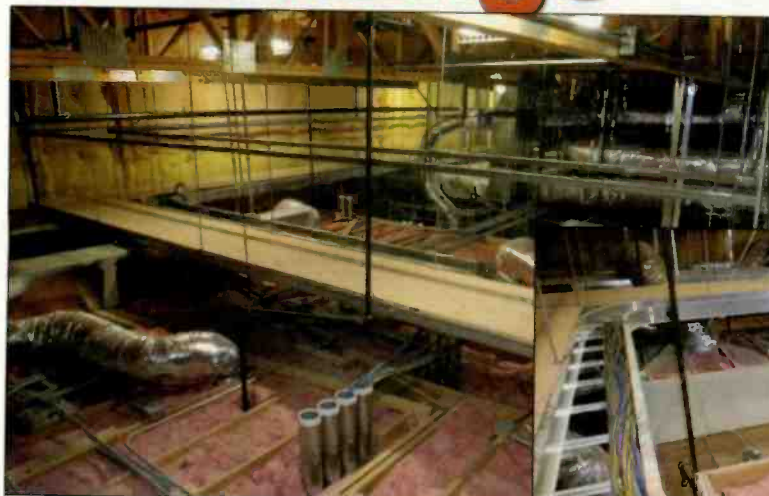
The catwalk built above the studios provides easy cable access.
