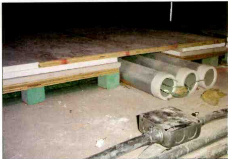
Cable conduits under the floating floor terminate at the hallway. Cabling runs under raised, removable hallway panels on the way to the machine room.
