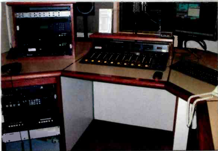
Control West: A typical setup for all four control rooms. The back panel under the Logitek ROC 10 is removable to access cabling and the punch block.
