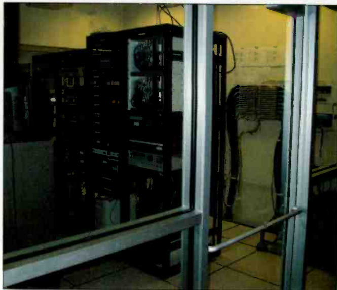
A view into the machine room. The glass panels were chosen for easy viewing as well as for "wowing" visitors.
