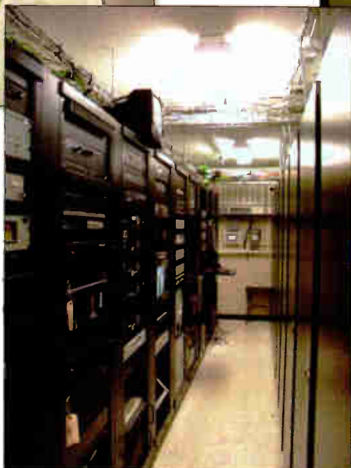
The tech center has two rows of racks. Instead of a wiring wall, trunk cables for each studio terminate in the racks.
