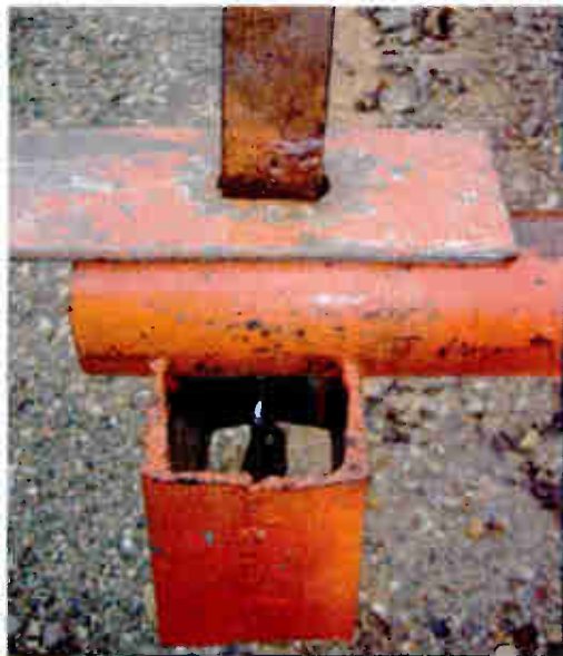
Figure 3. The padlock guard prevents the use of sledgehammer and bolt cutter to dismantle the lock. This is used on a gate that prevents vehicular entry.
