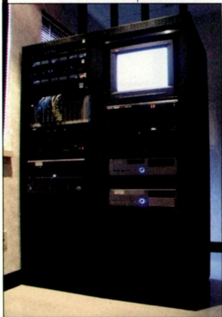
Even the smallest stations are able to leverage data technology in their facilities.
