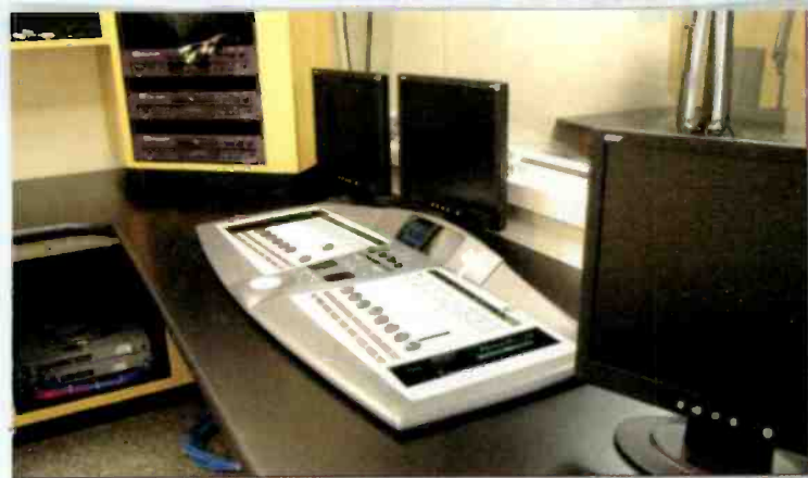
The facility is built around the Axia audio network. This is one of the control rooms.
